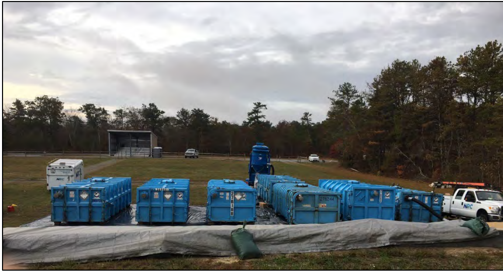
Photograph 2-5 Shows the vacuum and tight tanks for regrind removal.
