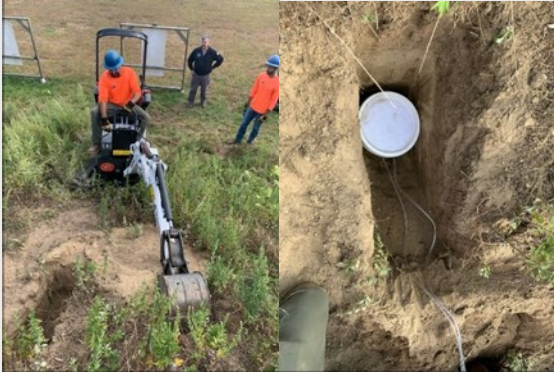
Lysimeter installation under a bullet pocket on the India Range backstop berm. Photos by MANG Environmental & Readiness Center
